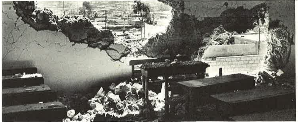
UNRWA's financial situation is aggravated by the necessity of repairing many schools, like this one in New Amman Camp, which were destroyed during the fighting last fall.
