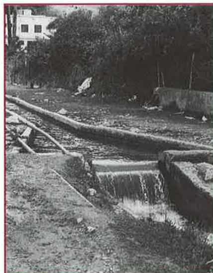
This antiquated irrigation canal, built in the 1930s, loses water by both evaporation and leakage.
