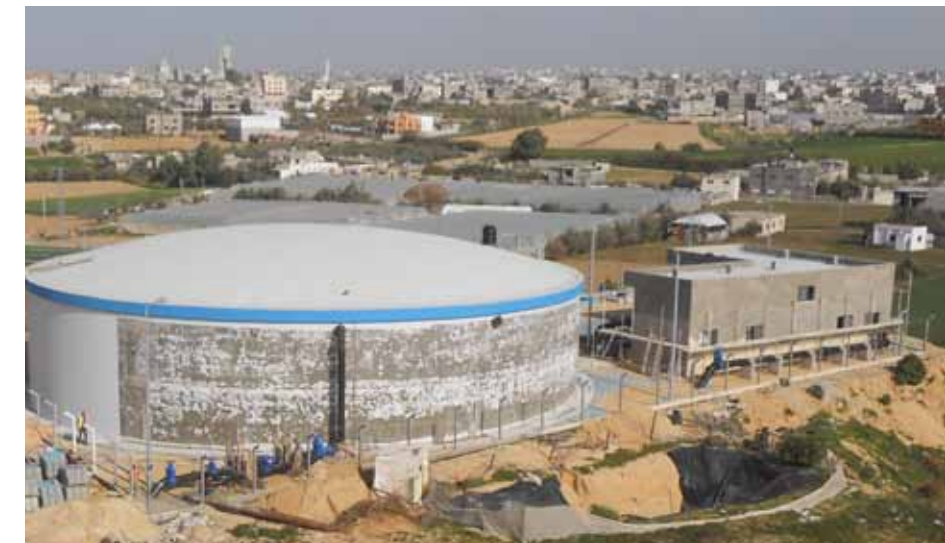
ANERA has nearly completed this 1.32 million gallon (5,000 cubic meters) reservoir and pumping station in southern Gaza, close to Khan Younis. It is the first of its kind to be built in Gaza in recent years.
